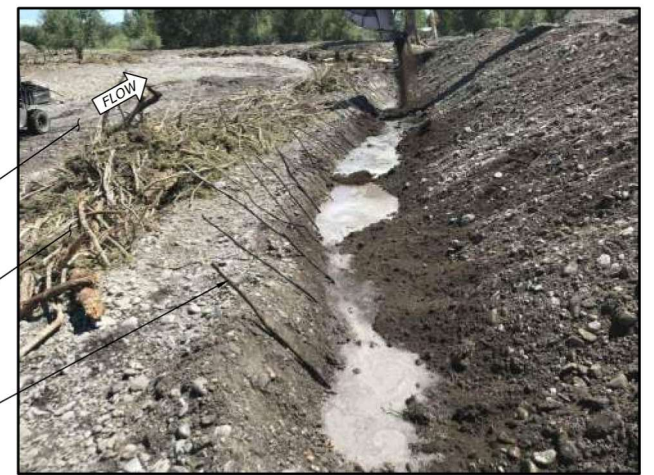
STAGE 1: MUD SLURRY IN BOTTOM OF EXCAVATED TRENCH WITH LIVE CUTTINGS PLACED.
