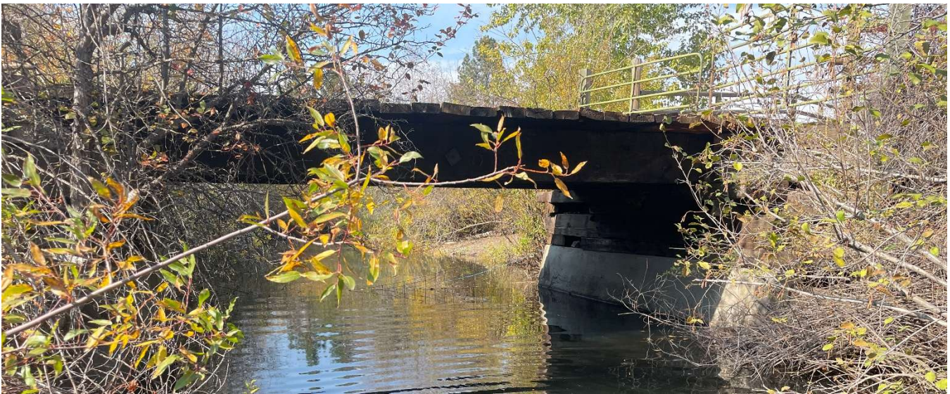
Figure 5-2. The lower timber bridge (looking downstream) is narrower than the channel width upstream and downstream of the crossing and shows signs of being flanked during high flows.
