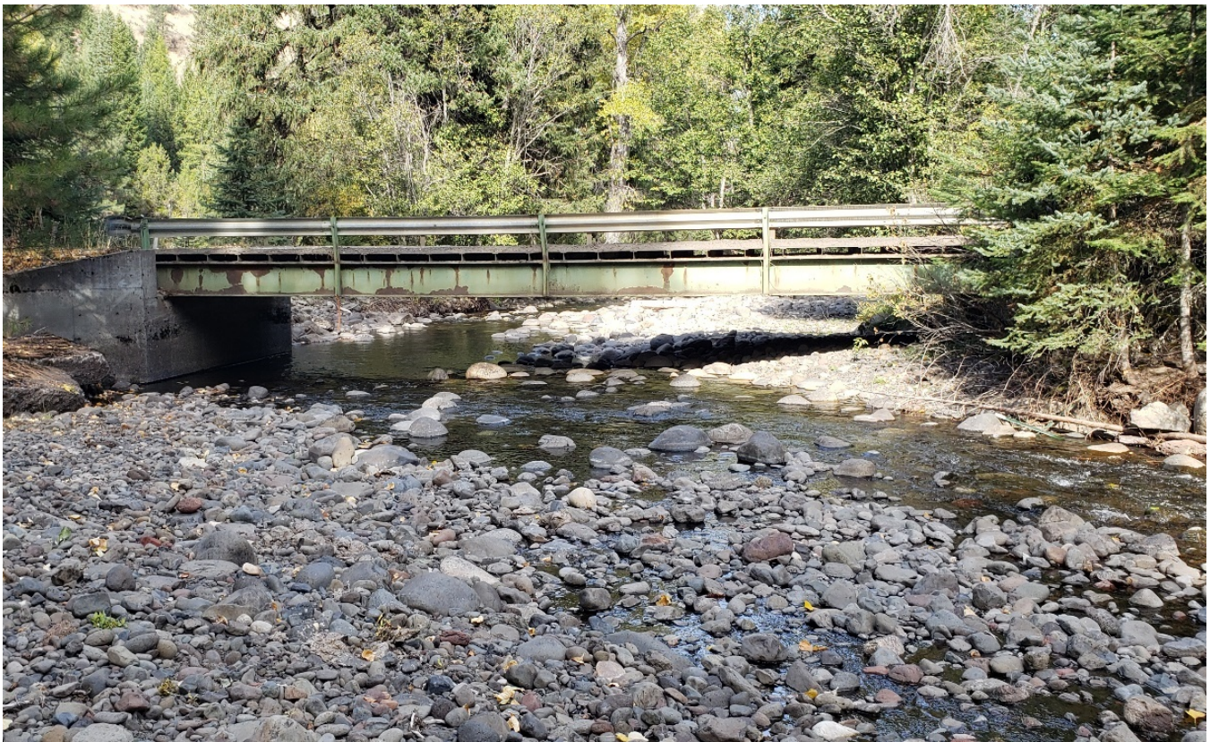
Figure 3-9. The existing Wallowa County bridge is located halfway through the project at RM 4.3.
