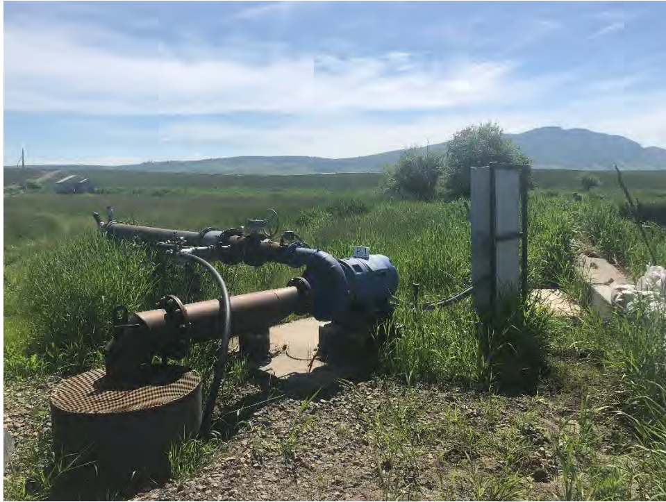
Pump 1 with electrical panel facing south
