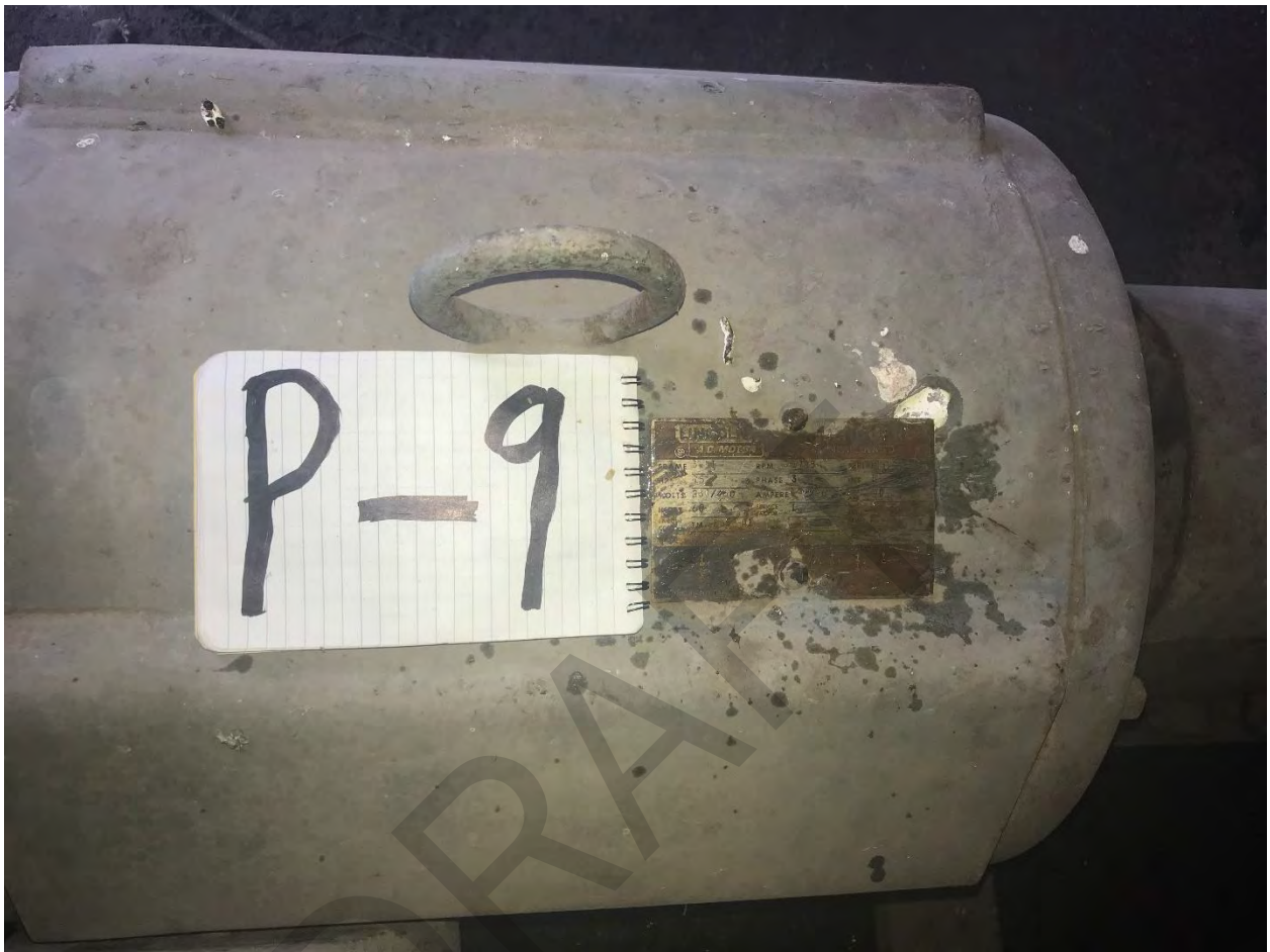
Pump 2 motor - 75 horsepower (Previously referenced as Pump 9)
