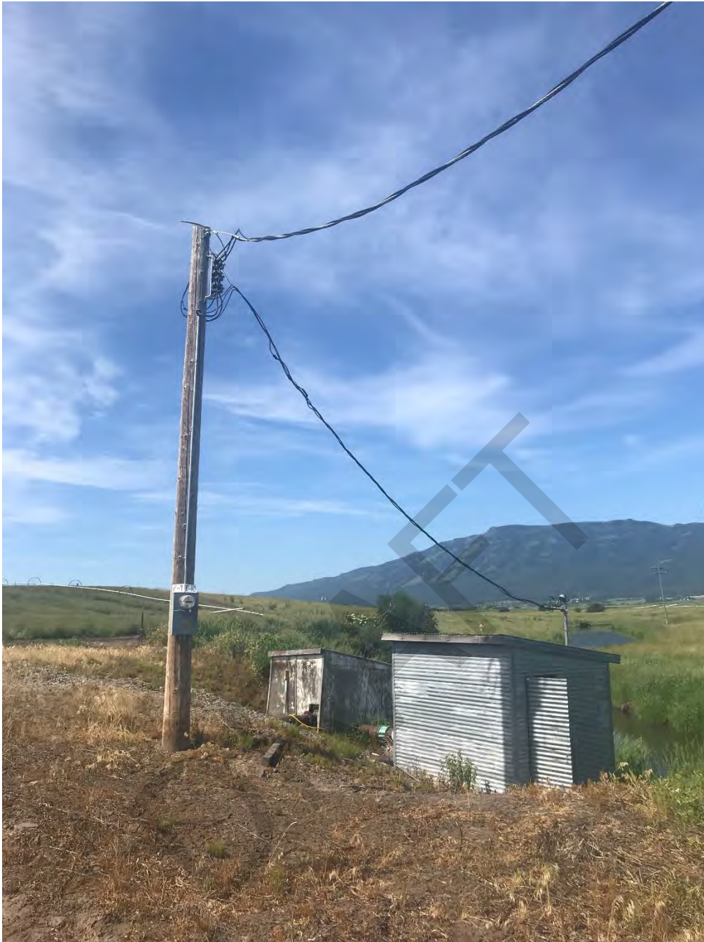
Pump 2 (foreground) and pump 3 (background) – facing south (upstream)
