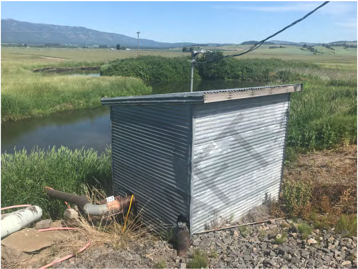
Pump 2 housing facing northwest (downstream)
