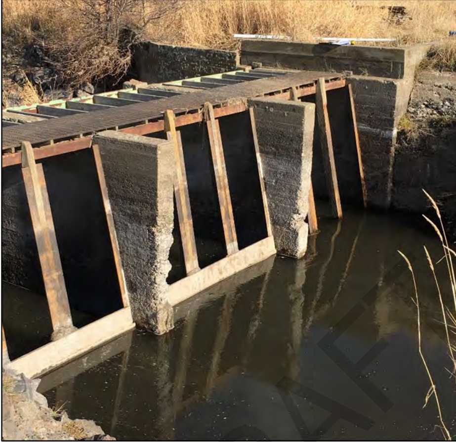
Photo 1. Existing stop-log operation of Royes Dam facing east, Willow Creek flows from right to left
