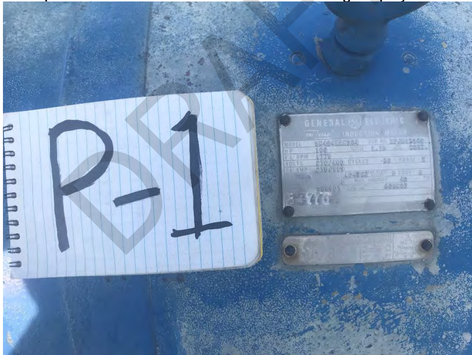
Pump 1 induction motor
