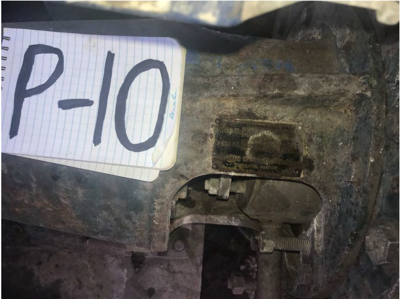
Pump 3 (Previously referenced as Pump 10)
