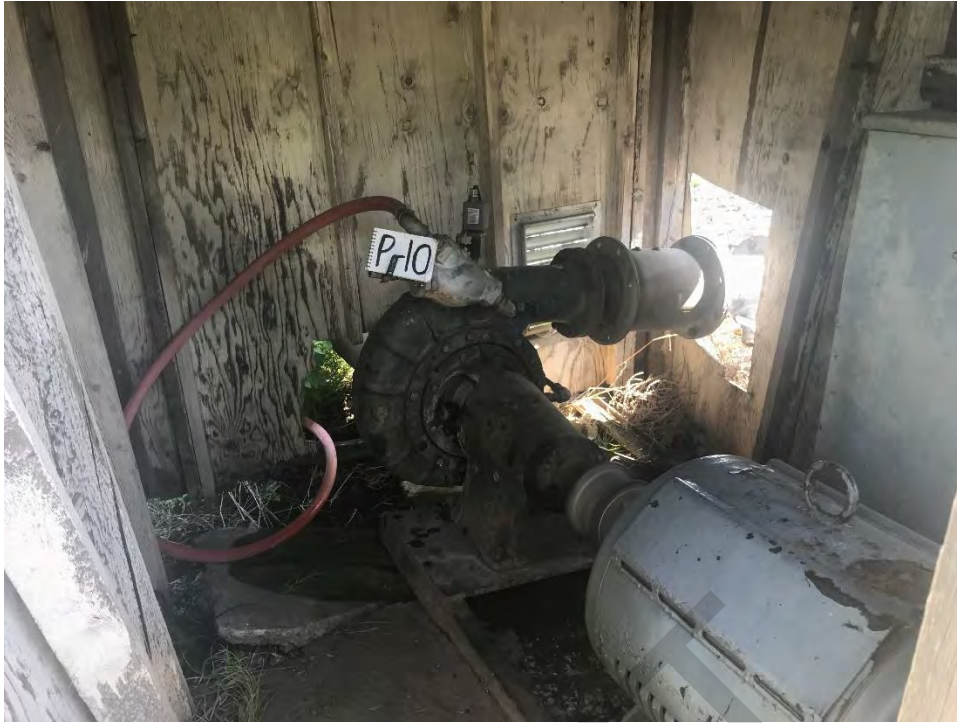
Pump 3 and motor (Previously referenced as Pump 10)
