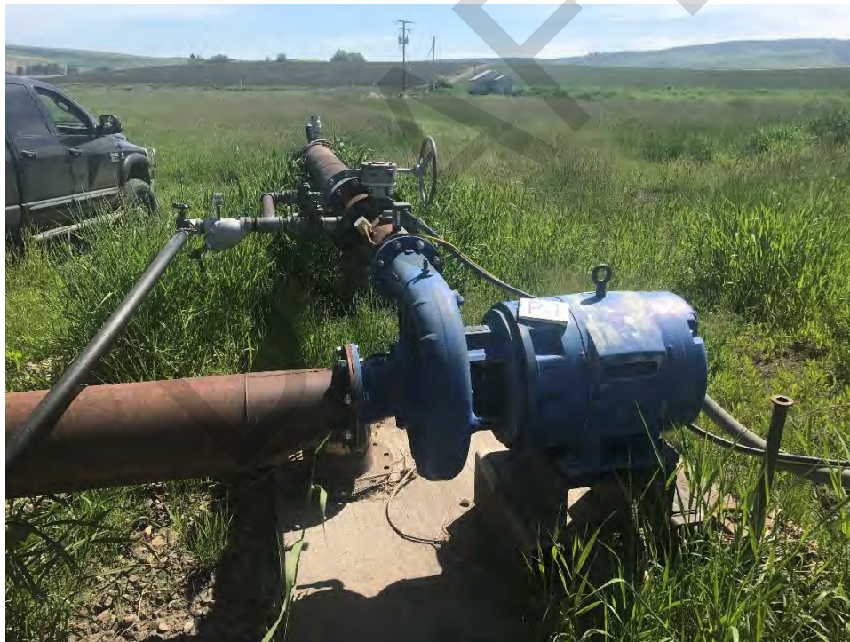
Pump 1 with delivery pipe facing east
