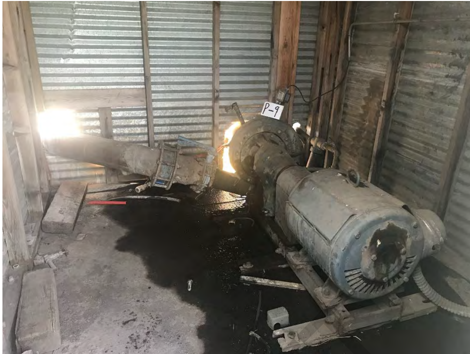
Pump 2 and motor - outlet pipe to the left
