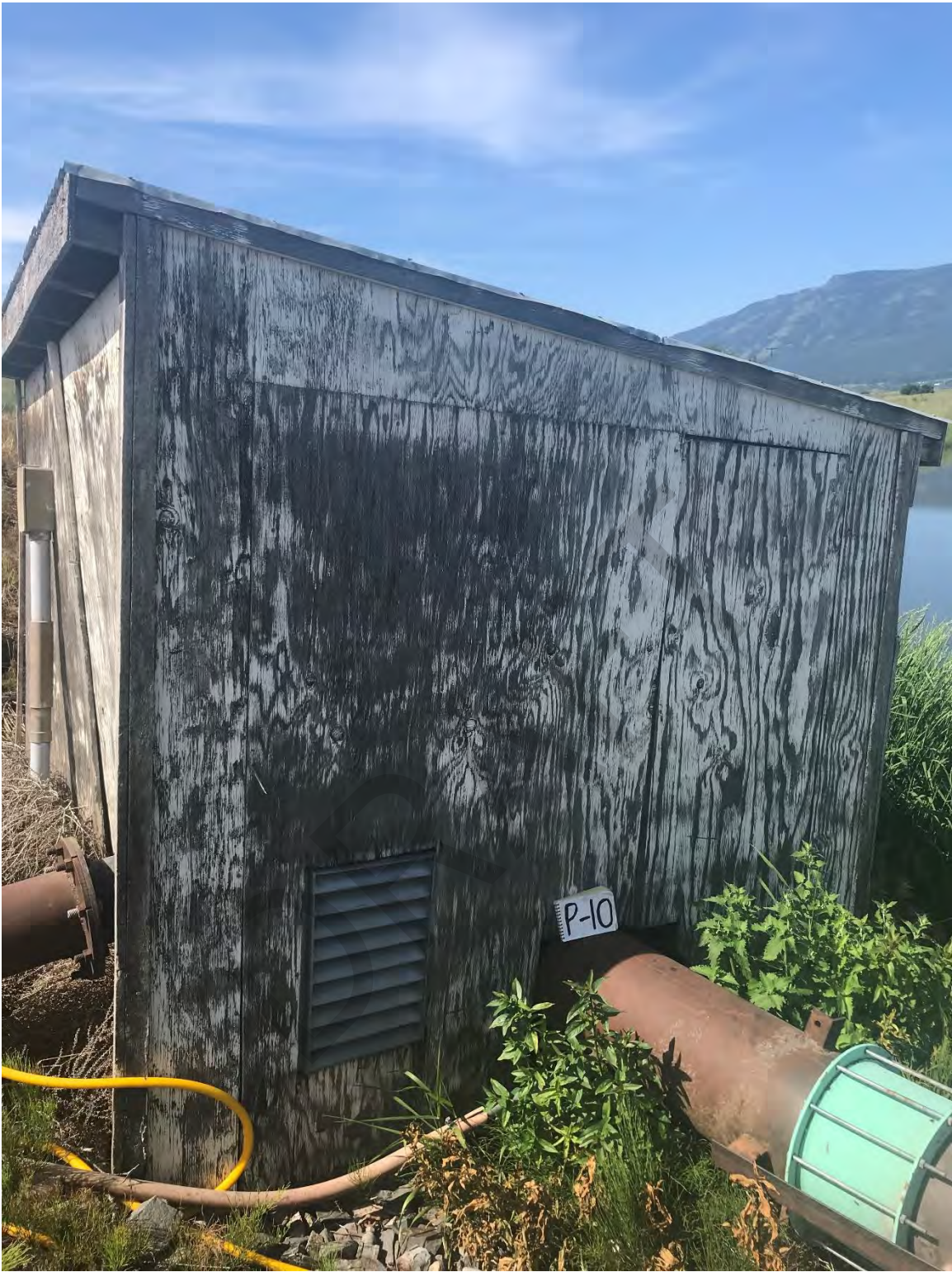
Pump 3 housing and intake pipe (right) outlet pipe (left) (Previously referenced as Pump 10)
