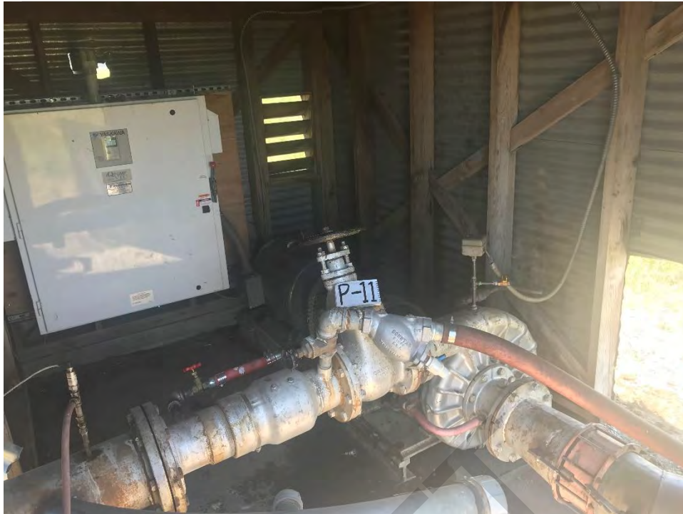
Pump 4 and electrical control panel (Previously referenced as Pump 11)
