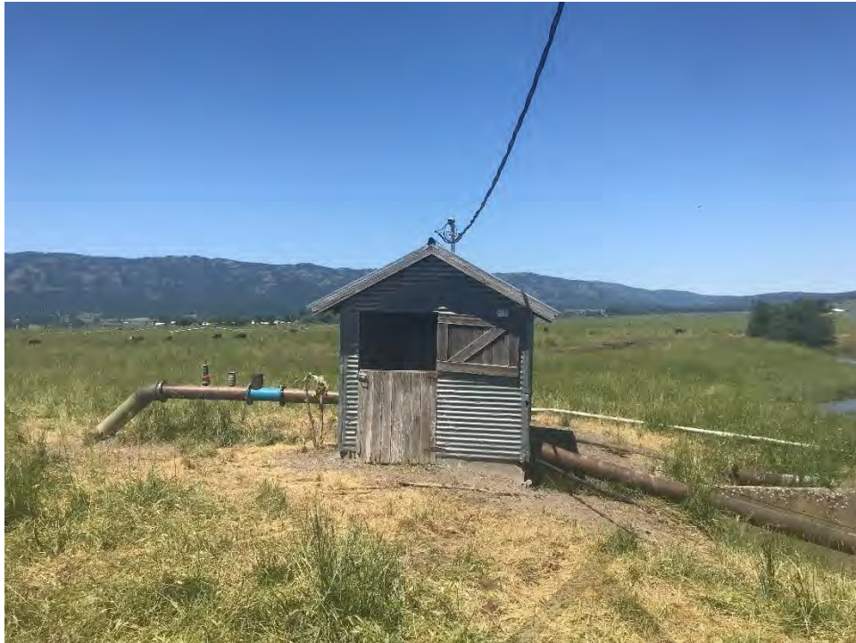
Pump 4 housing, intake right and outlet right, facing west (upstream)
