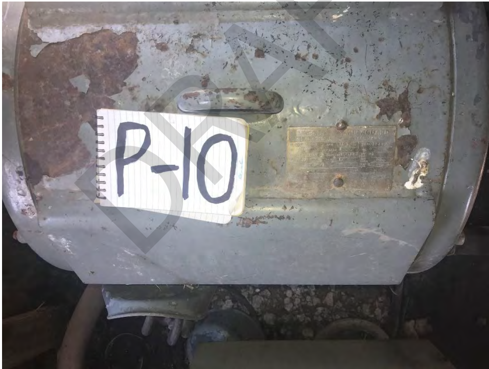
Pump 3 motor – 100 horsepower (Previously referenced as Pump 10)
