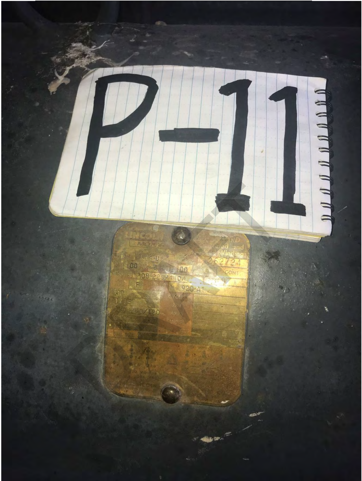
Pump 4 motor – 100 horsepower (Previously referenced as Pump 11)
