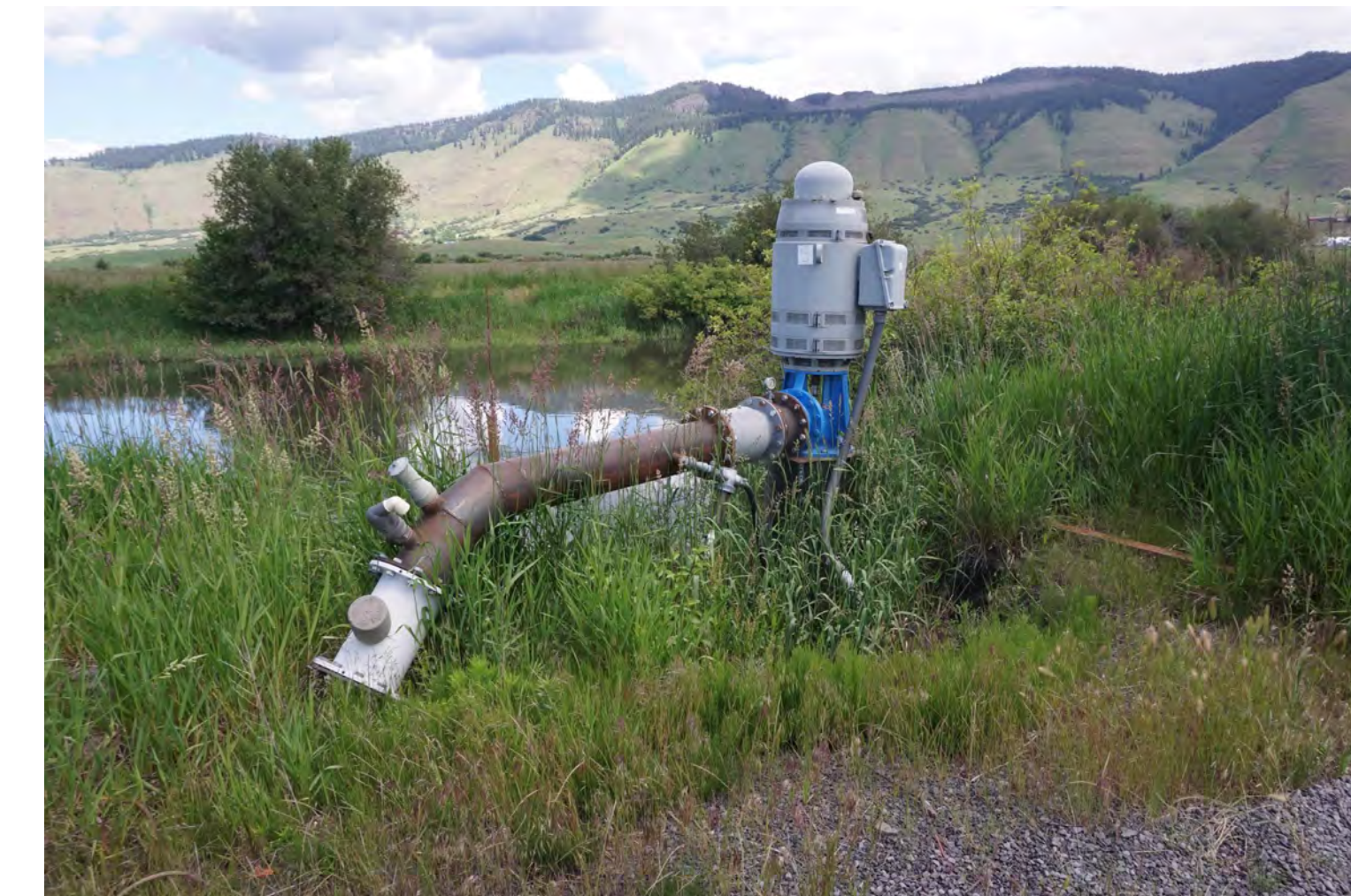
EXISTING VERTICAL TURBINE PUMP
