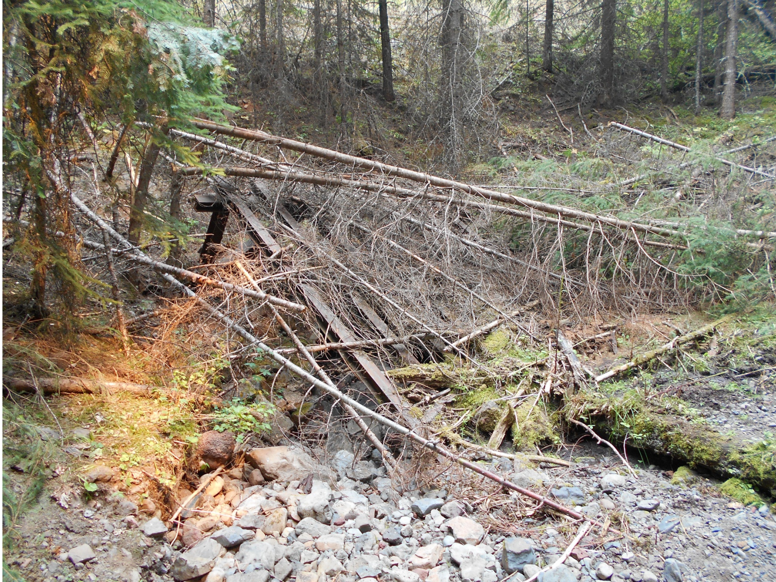
West Fork Broady Trash Rack and View Upstream
