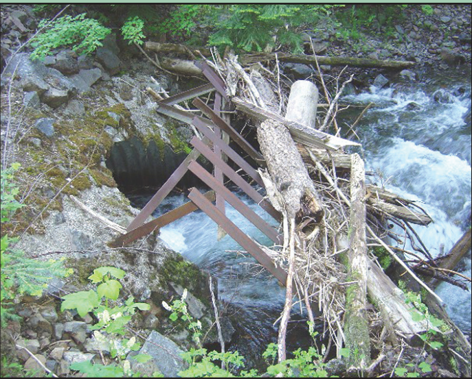
Photo 1: Pre-project photograph showing log weir in foreground and arch in background. The log weir presents a 3-foot jump height that precludes many juvenile fish from swimming upstream. During high flows, streamflow through the arch is fast enough to reduce passage for smaller, less able aquatic organisms.
