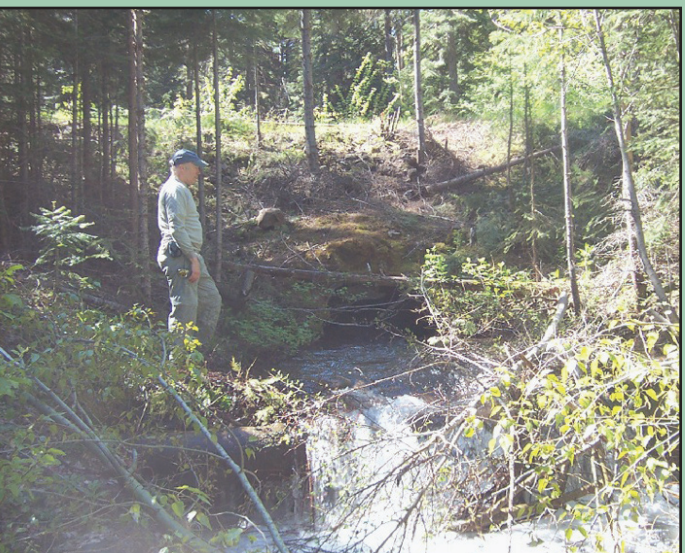
Photo 2: Pre-project photograph showing log weir in foreground and arch in background. The log weir presents a 3-foot jump height that precludes many juvenile fish from swimming upstream. During high flows, streamflow through the arch is fast enough to reduce passage for smaller, less able aquatic organisms.
