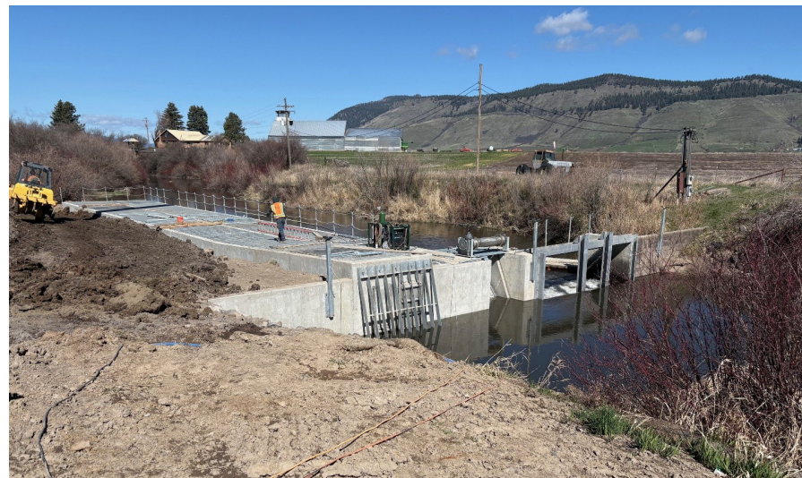
Nearing completion of the new fishway with installation of an overshot gate and steel stanchions in Elmer Dam.
