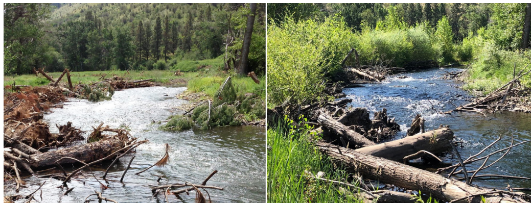
Left: 2016, immediately post-construction with newly placed large wood. Right: 2019, showing persistent wood complexity, rapid vegetation recovery, and deep pool development. (Courtesy of the CTUIR)
