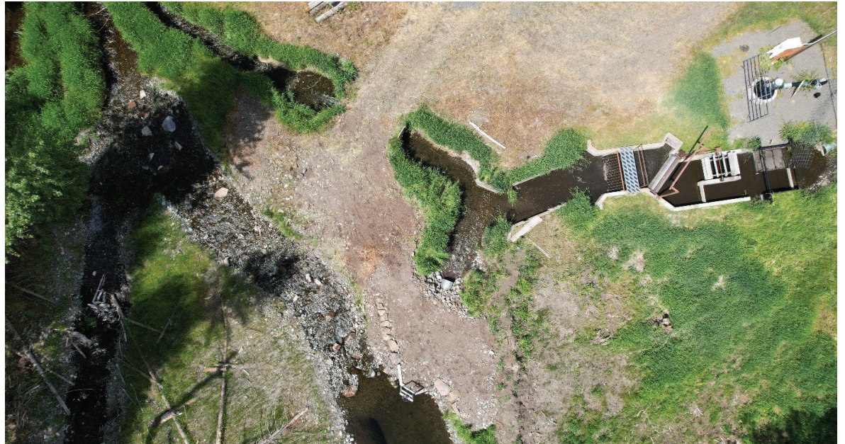
An aerial photo of the completed project showing the new roughened riffle, the installed headgate, utilization of the existing ODFW fish screen, and the relocated pivot pump and sump. (Photo courtesy of GRMW)
