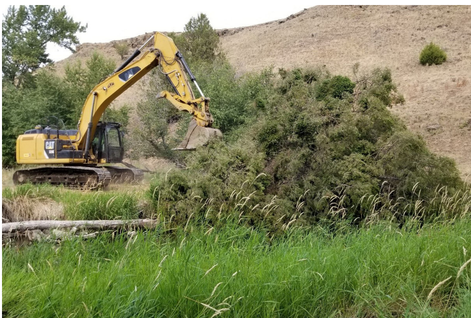
An excavator operator places a juniper tree that will become part of a large wood structure. Photo by Winston Morton, ODFW.
