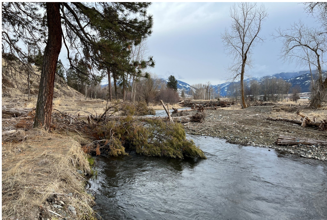
A whole juniper tree placed in the river, creating slow water for juvenile fish to rear and ideal spawning conditions from gravel that has dropped out in the slower water. Photo by Ian Wilson, GRMW.
