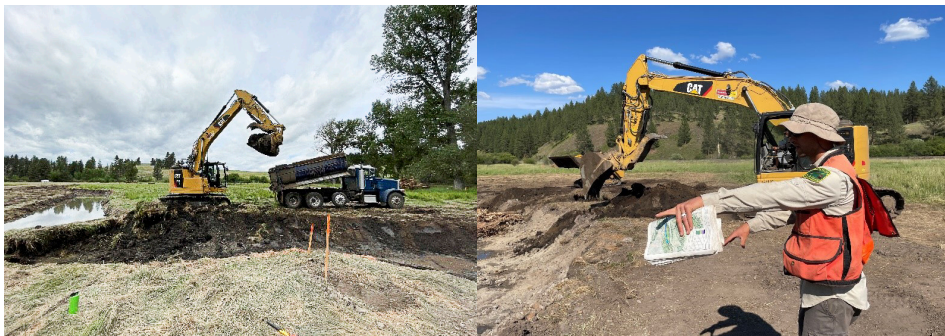
On the left, Northwest Watershed Restoration, the contractor hired to assist with implementation, constructing a side channel. On the right, ODFW Fish Habitat Biologist Nick Smith planning the next wood structure layout. (courtesy of ODFW)
