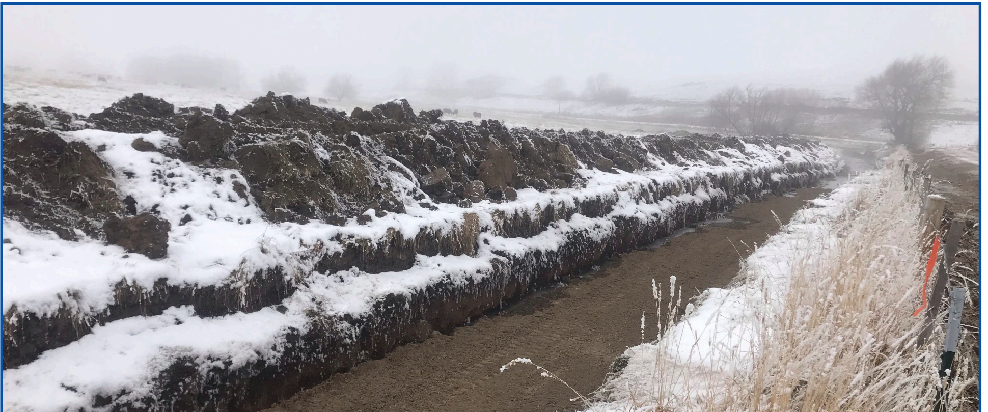
A section of trench that is prepared and ready for pipe installation. The Farmers Ditch, which the new pipeline will replace, is visible on the hillside in the distance. The ditch will be kept intact to serve as a catchment area and wildlife habitat (courtesy of GRMW).
