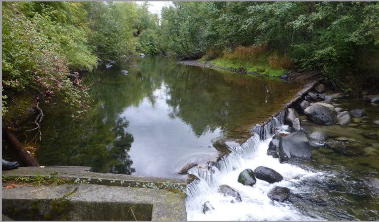
The Sheep Ridge diversion structure on the Lostine River before restoration was completed by the Nez Perce Tribe and GRMW (courtesy of Katie Frenyea).
