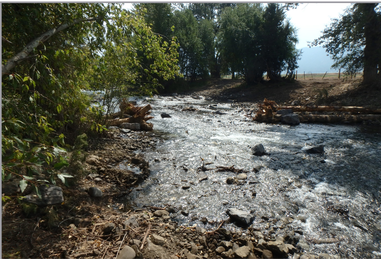
After the Tulley Hill restoration was completed in 2017. Passage for juvenile fish was restored while still maintaining access for irrigators (courtesy of Katie Frenyea).
