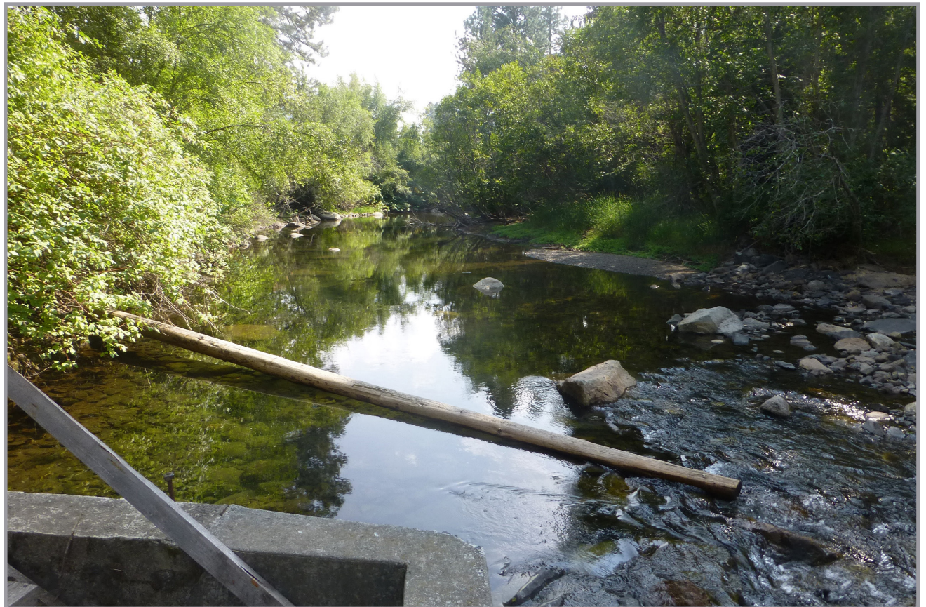
After the Sheep Ridge diversion structure was removed and restoration was completed in 2016. This project restored passage for anadromous fish to prime spawning habitat (courtesy of Katie Frenyea).
