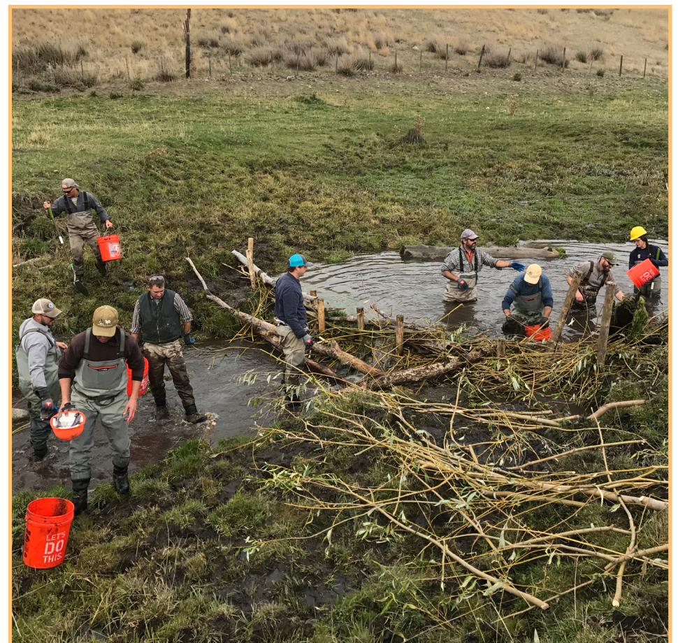
After BDA installation: ponded water has lifted the logs that were embedded in the stream bottom. This log was later used upstream in a post-assisted log structure (courtesy of GRMW).
