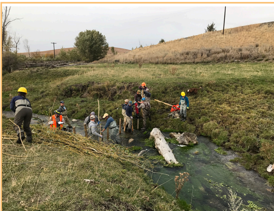
BELOW: Participants work to drive posts, and prepare for creating a willow weave (courtesy of GRMW).
