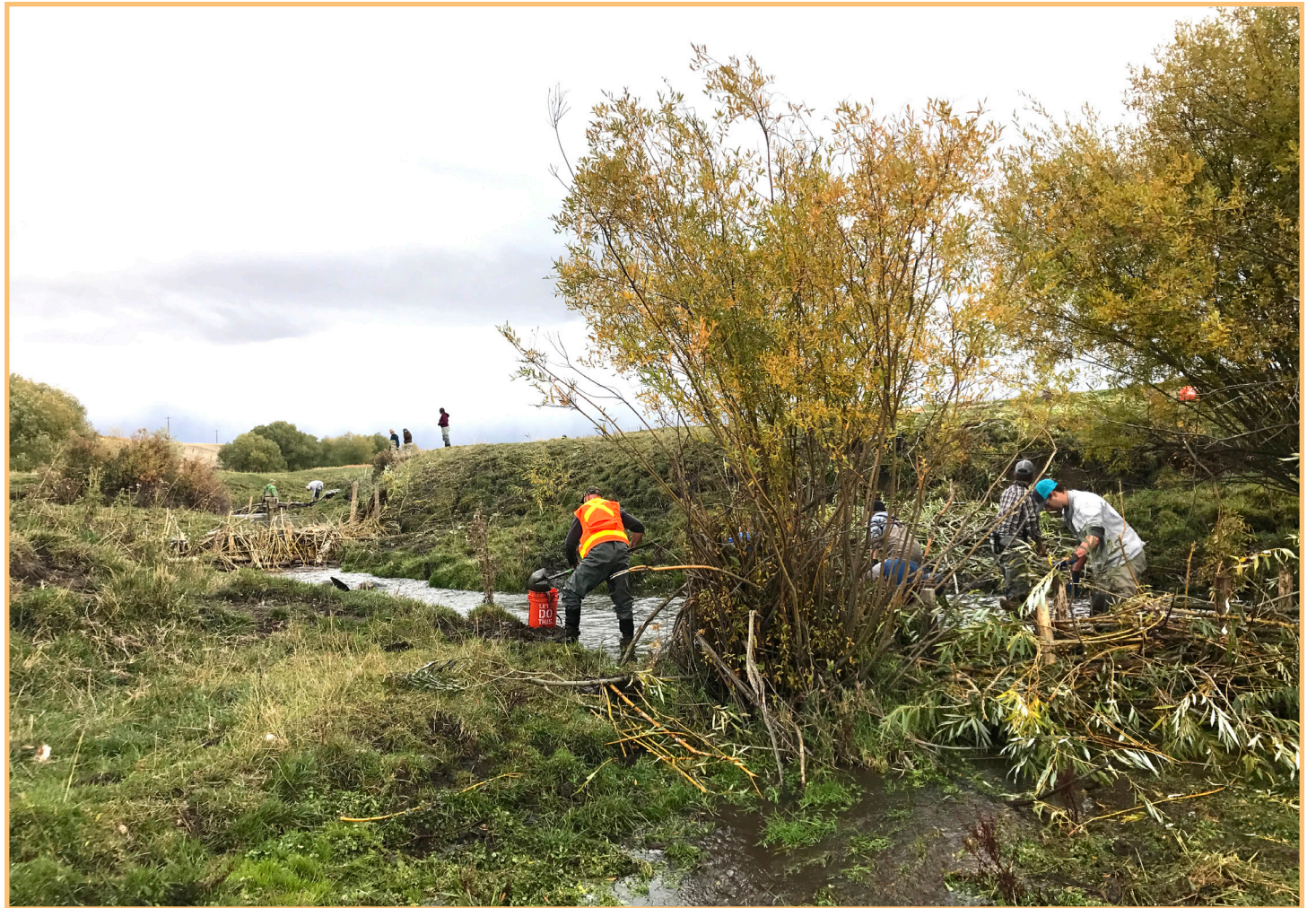
Workshop attendees build a second BDA downstream of the primary dam. Upstream attendees work on building a post-assisted log structure (courtesy GRMW).
