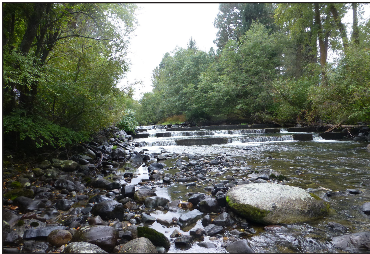
Looking upstream at the deteriorating concrete walls that no longer meet fish passage criteria, and the wooden check dam that makes fish passage difficult during low flows. This photo was captured from below the fishway and diversion for the Sheep Ridge irrigation ditch.
