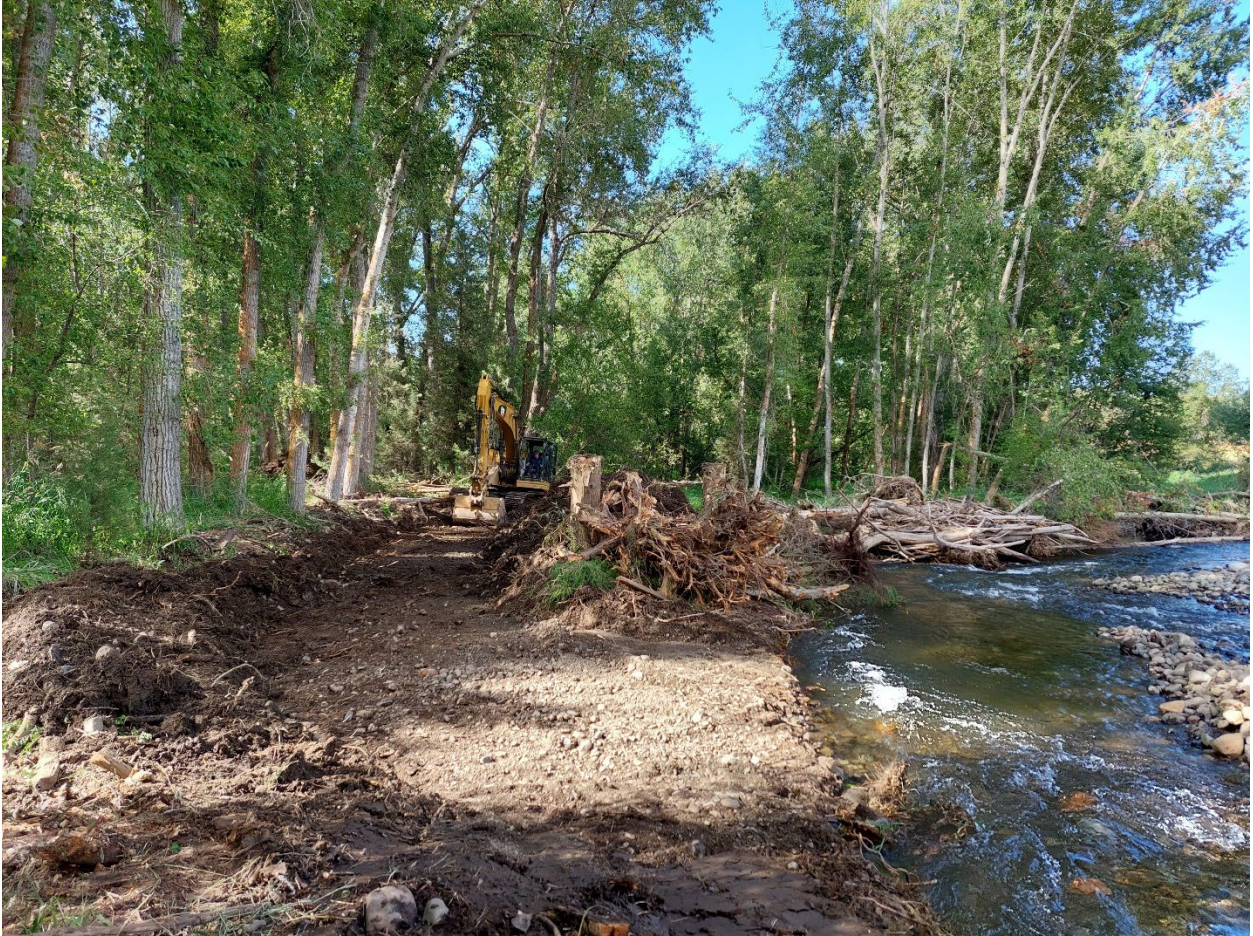
Figure 4. Finishing up grading behind completed Small Apex Jam in Pilot Channel Inlet 2, taken 8/4/22.
