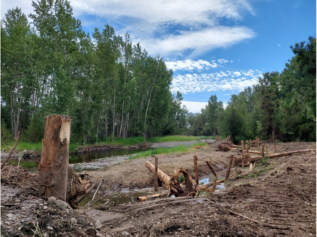
Figure 3. Completed Alcove 1 including two Small Apex Jams and four Vertical Post Arrays, taken 8/4/22.
