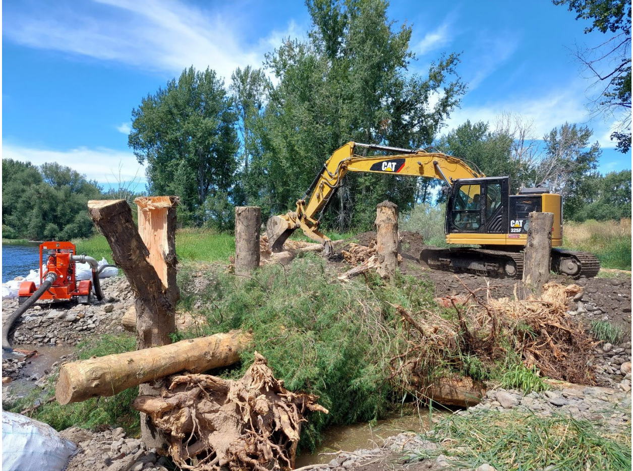
Figure 1. Installation of Large Apex Jam A1 adjacent to Pilot Channel 1 Inlet, taken on 8/2/22.
