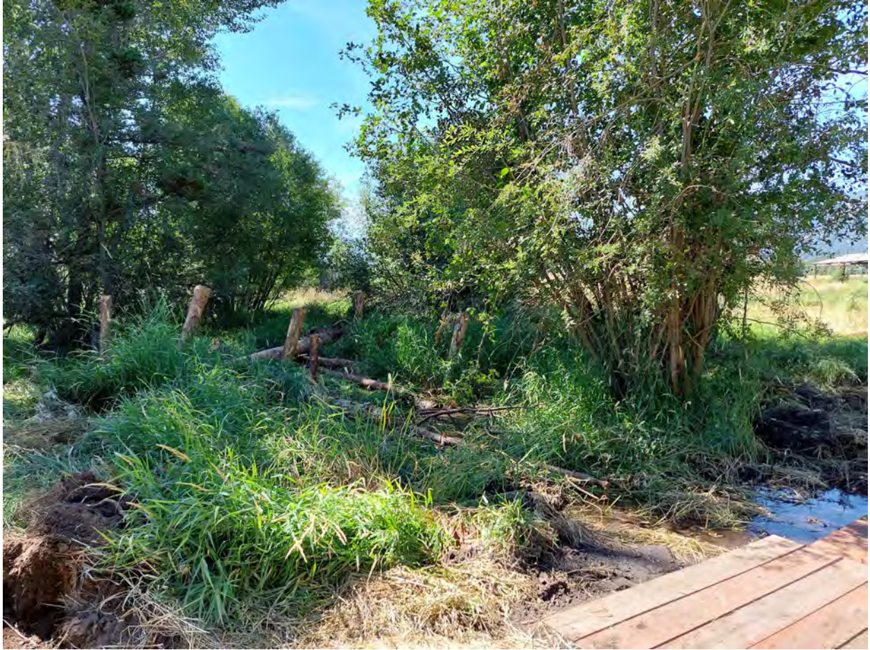
Figure 4. Vertical post array installed in floodplain swale, taken during construction on August 5.
