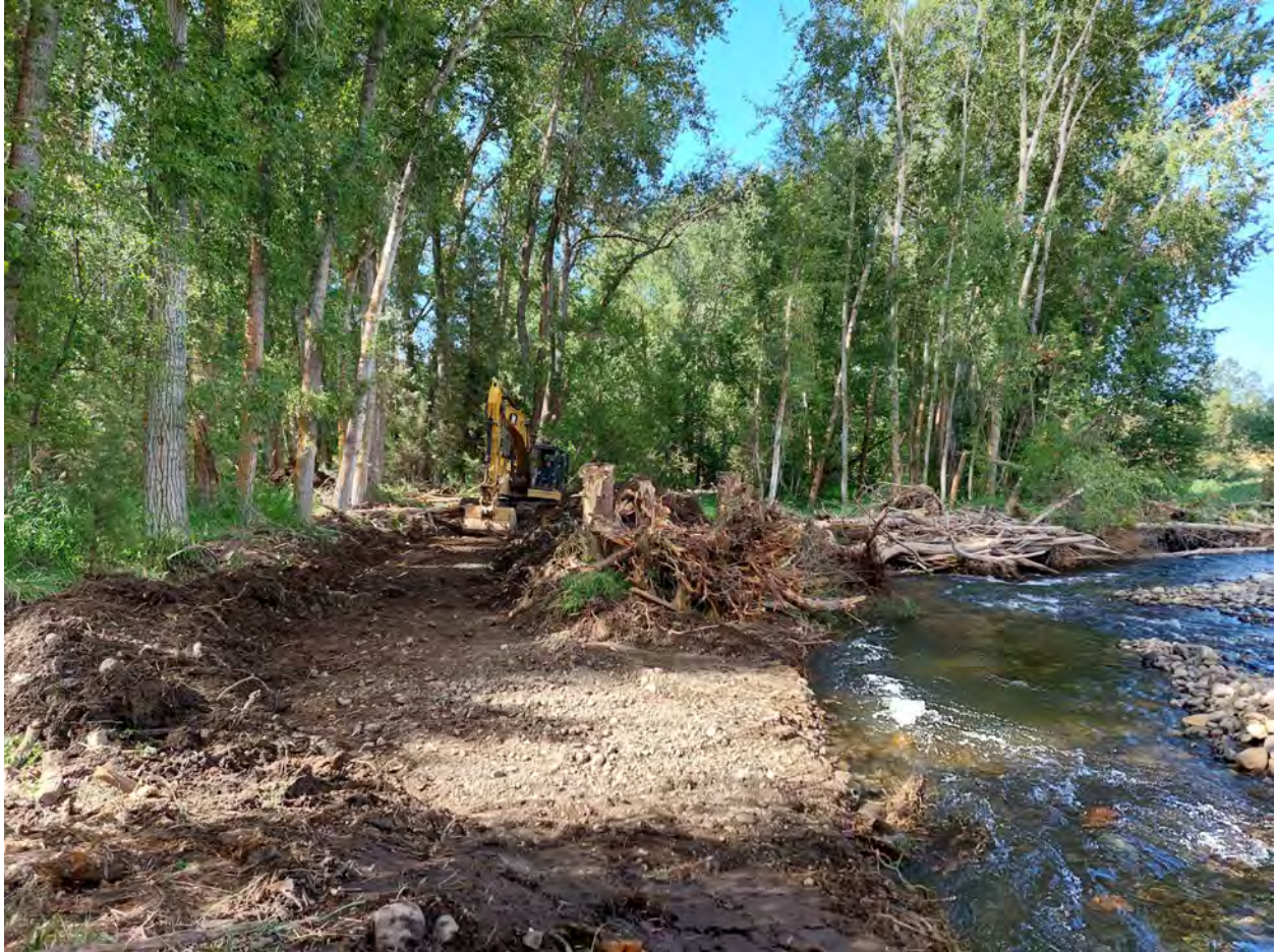
Figure 3. Looking downstream from river left at Pilot Channel 2-Inlet grading and associated small apex jam, taken during construction on August 4.
