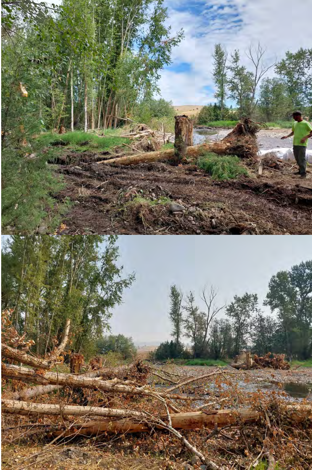
Figure 6. Looking toward Losine River at Small Apex Jam in Pilot Channel 2-Inlet during construction (top) and after windstorm wood addition (bottom).
