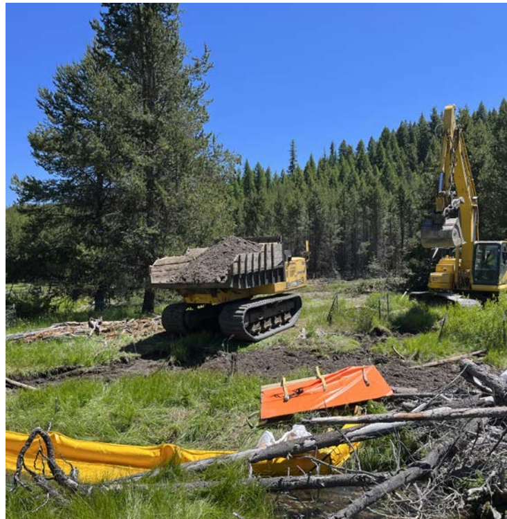
Photo: This photo shows the construction operators hard at work in the 2023 construction season.
