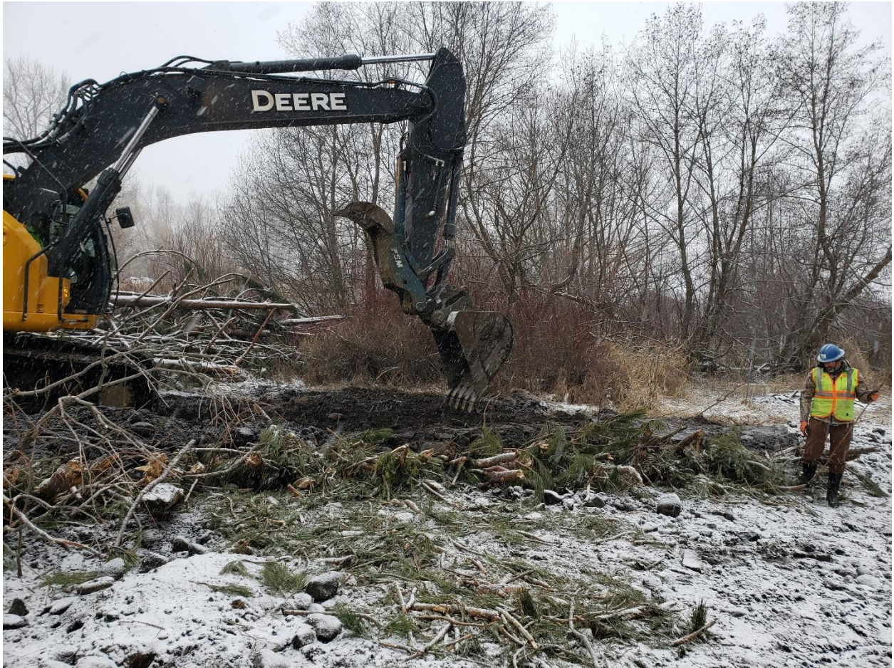
Figure 3. Brush bank treatment installation left bank in downstream extent of SC1, taken 2/11.
