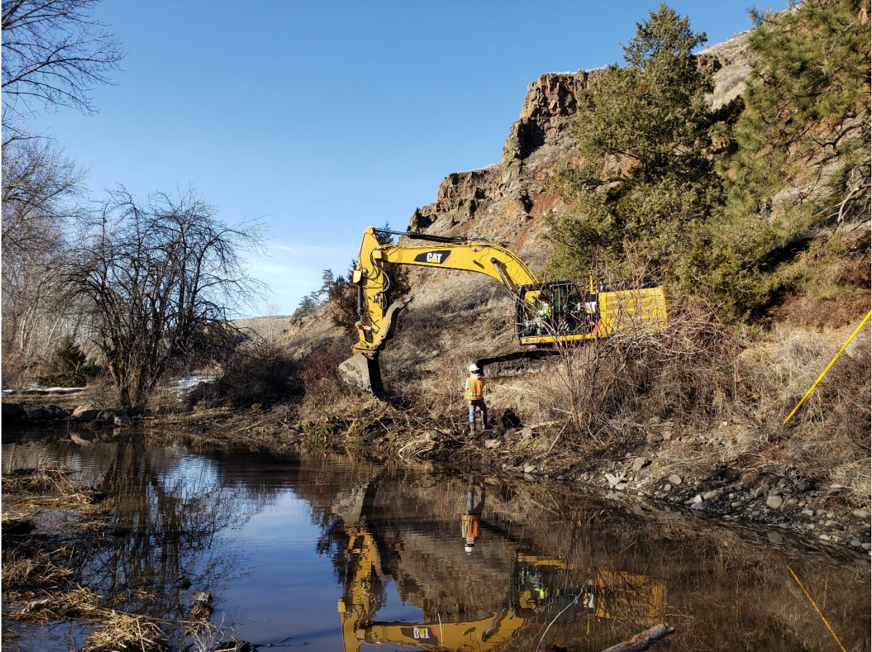
Figure 2. Modified willow trench install in downstream right bank of alcove in SC1, taken on 3/3.
