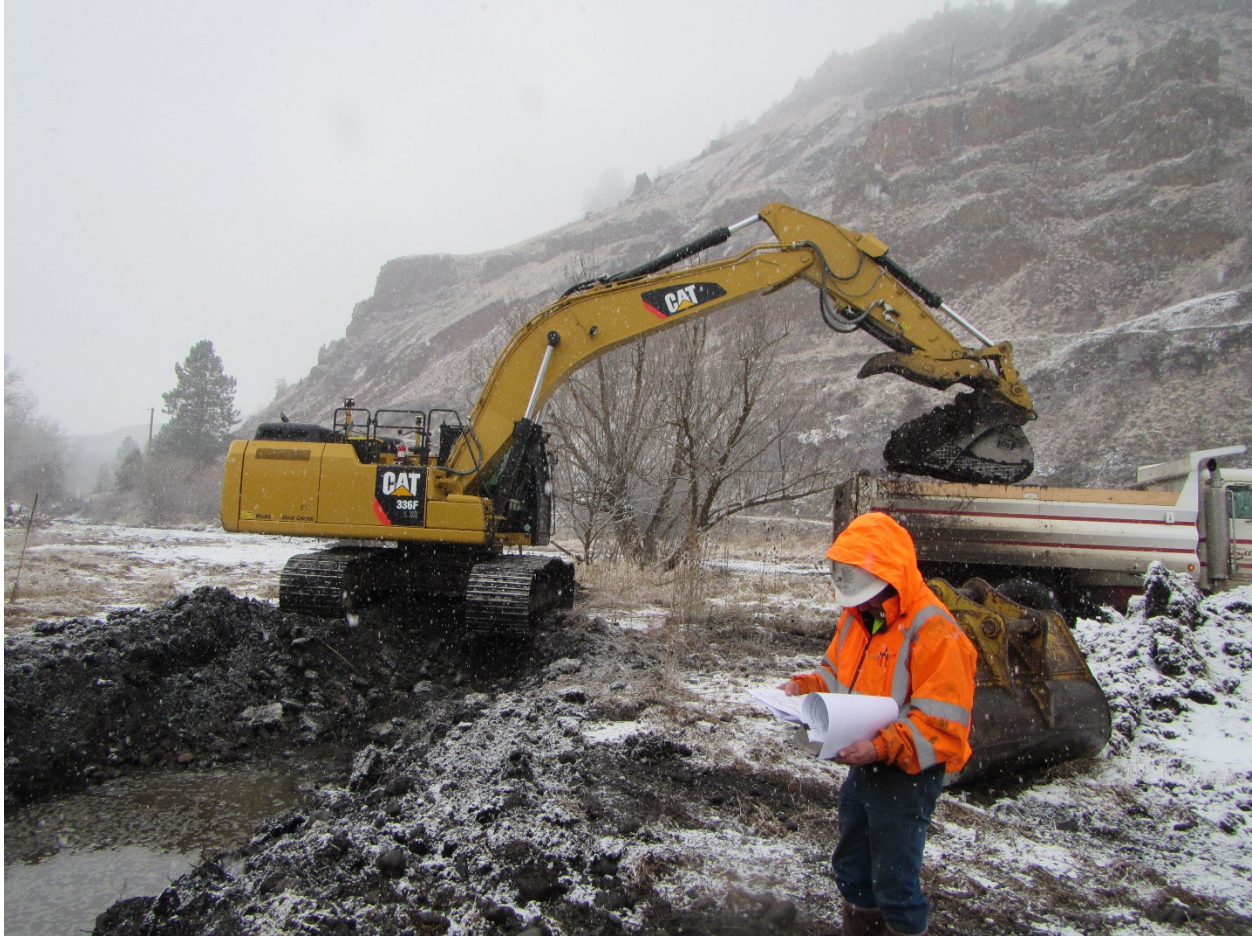
Figure 2. The CAT 336 excavating downstream in SC3 and placing fill material (general fill) in the end dump for haul off site.
