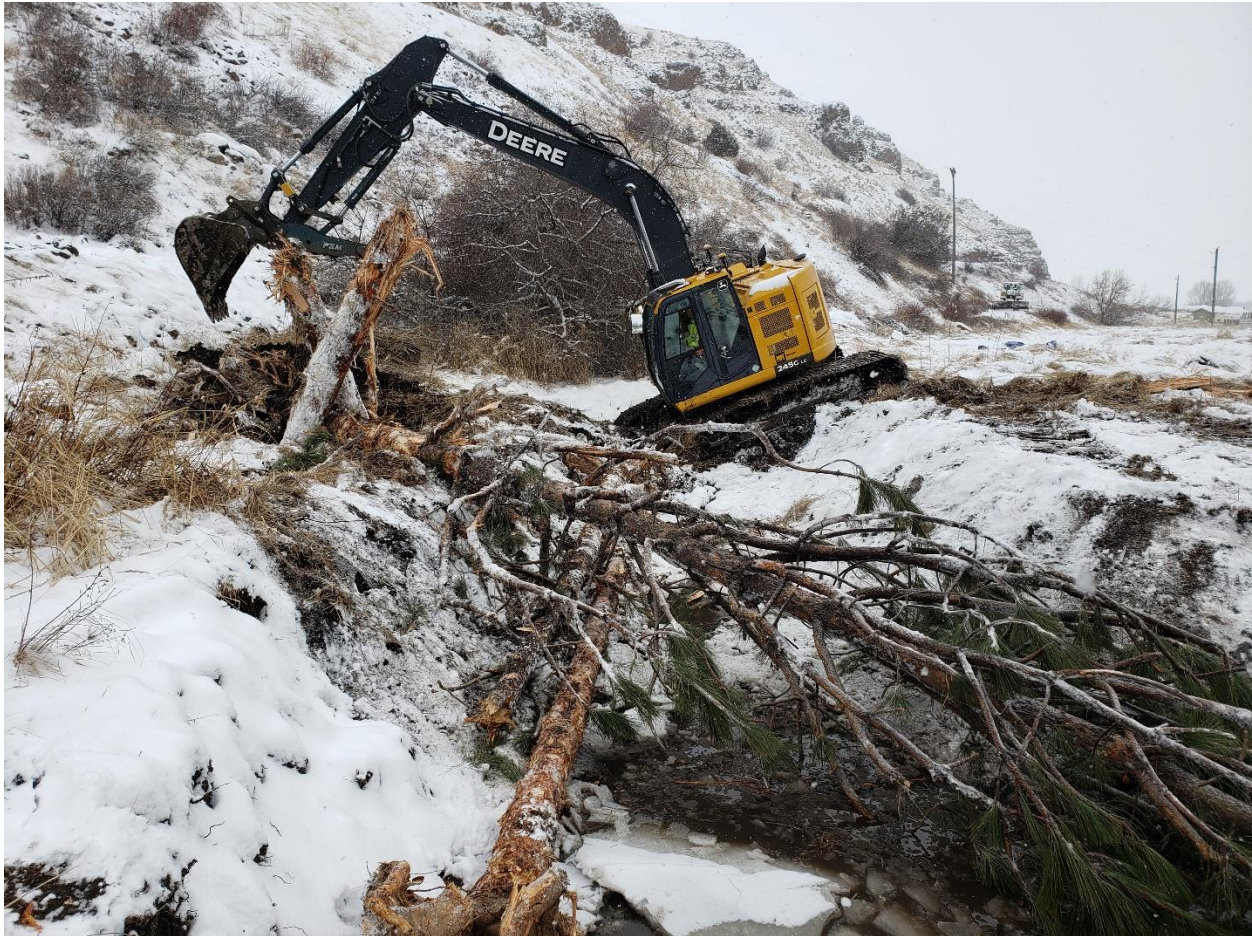
Figure 4. Installation of alcove whole tree habitat structure and associate pilings (~Station 8+75), taken 2/12.
