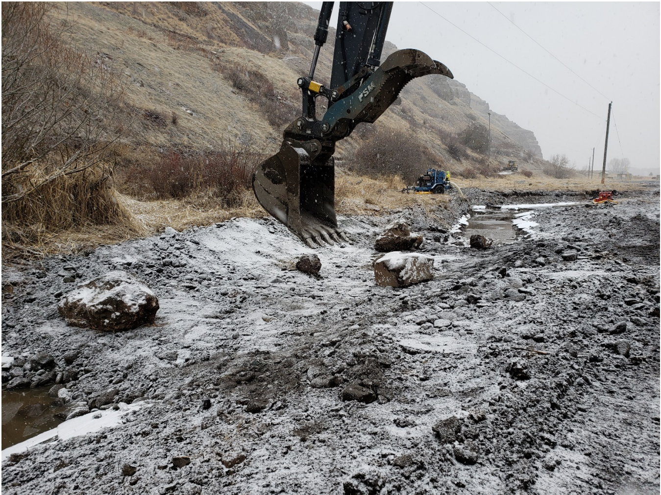
Figure 3. A fish screened pump is shown pulling water out of side channel 1 during downstream riffle construction on 2/11/21.
