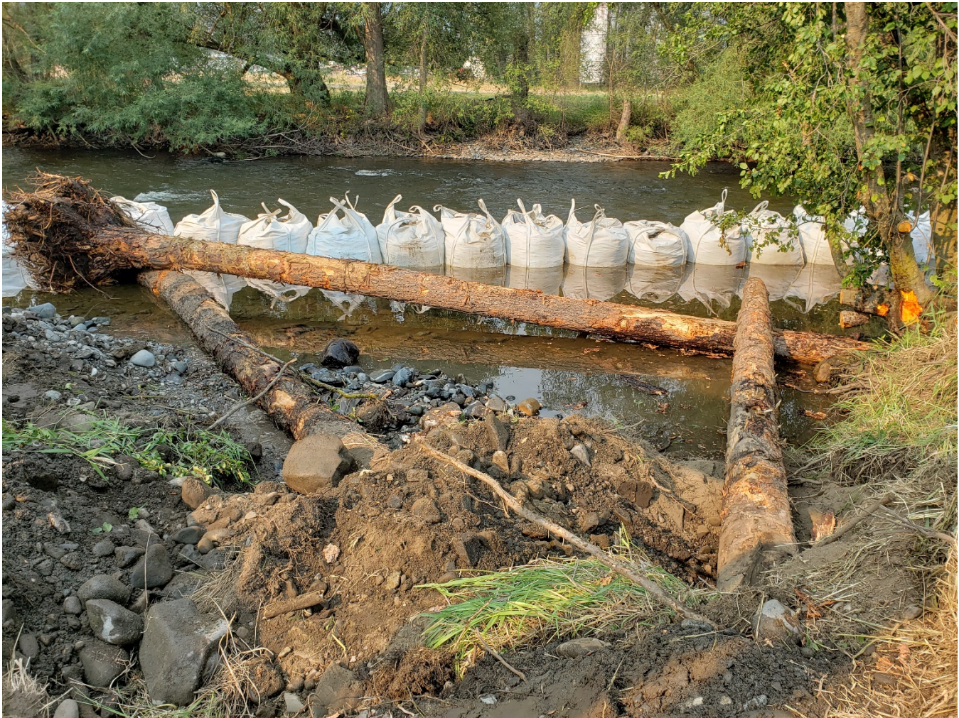
Figure 6. Super sack/sheet plastic work isolation area at channel 1 inlet and Wallowa River mainstem (8/3/21).
