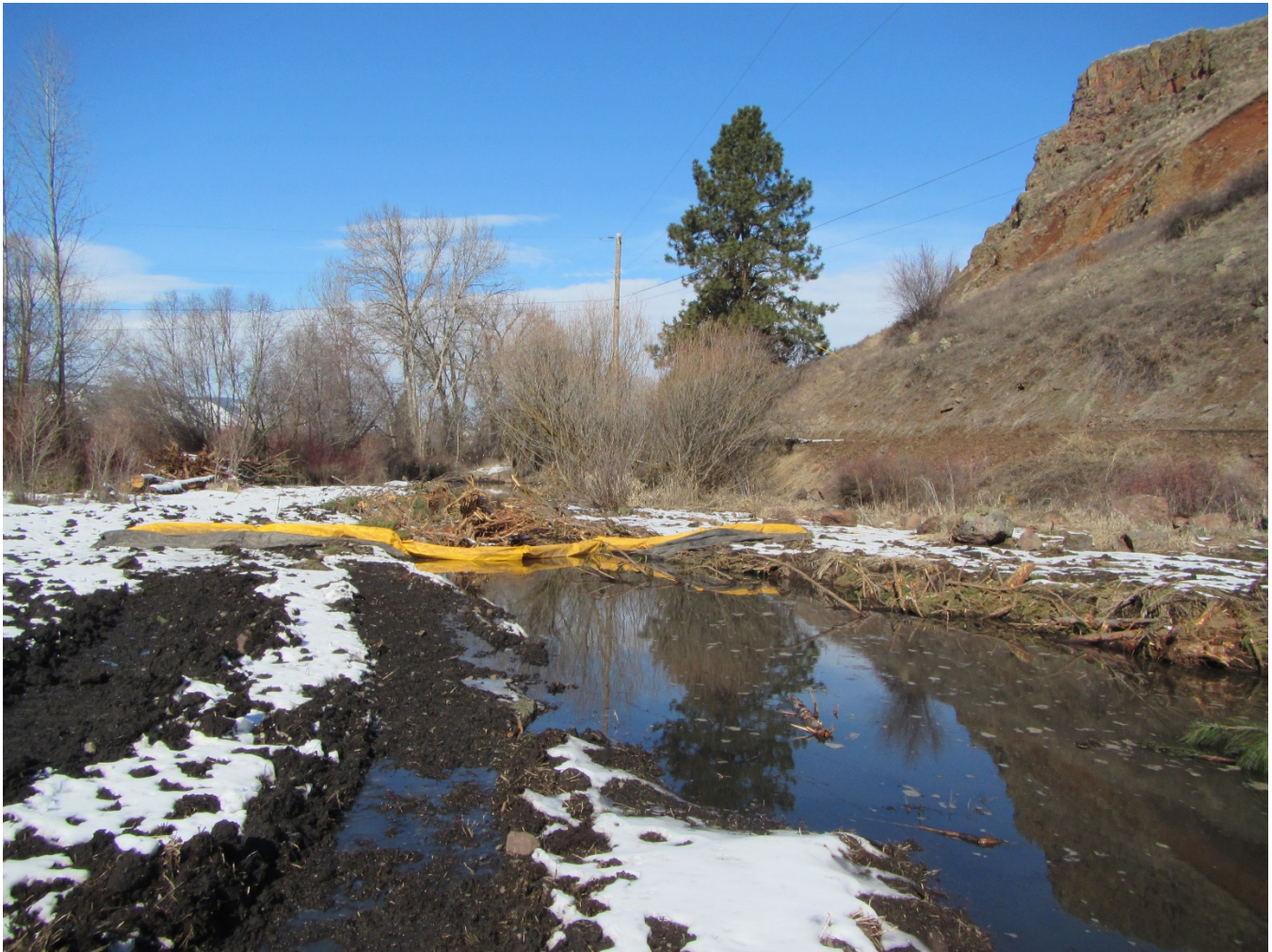
Figure 5. Silt fence placed downstream of side channel 1 and 3 confluence, upstream of alcove (3/2/21).
