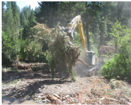
Racking material for stream
