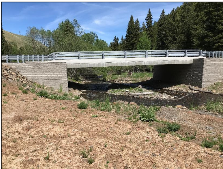
Photo 2: Top left: standing upstream of double culvert (2018). Stream substrate and debris aggrades at top end of culverts causing a jump height barrier to fish passage. Top right: Upstream view of new bridge and improved fish passage (2019) and bottom left (2021).
