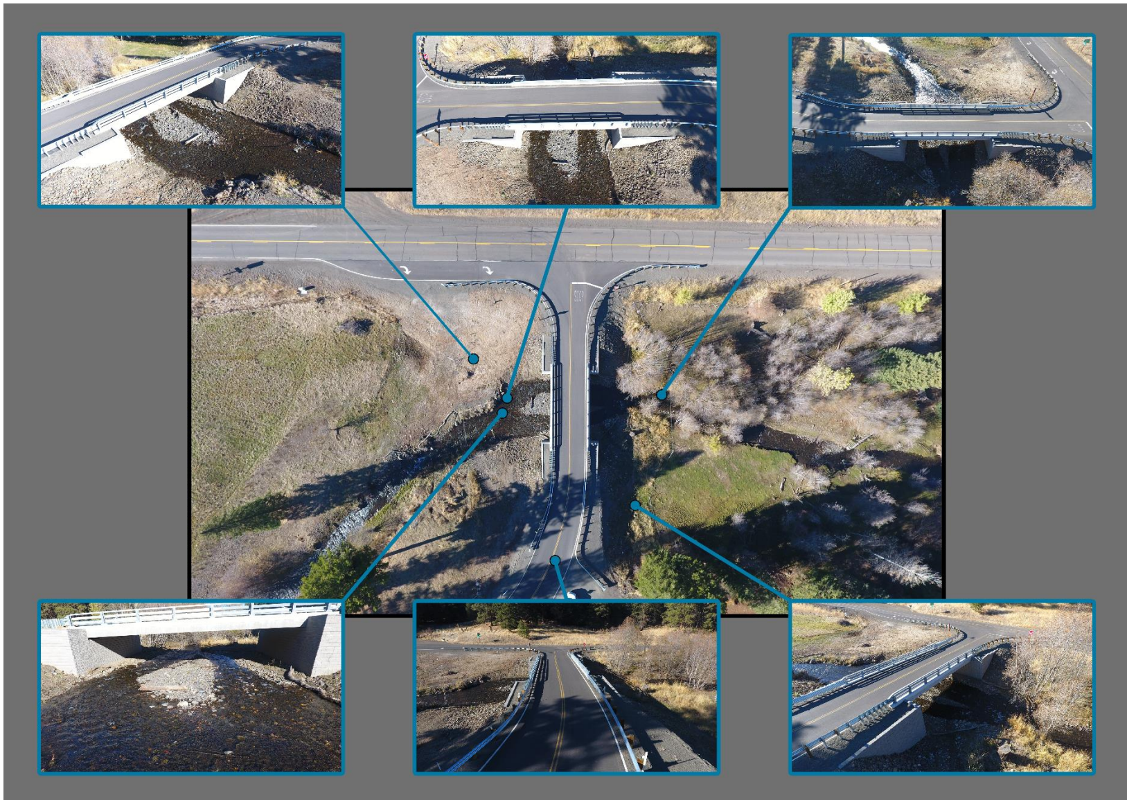
Photo 6. Drone imagery captured post project in 2020. The images show the improved sediment transportation and sorting as well as the new bridge alignment.
