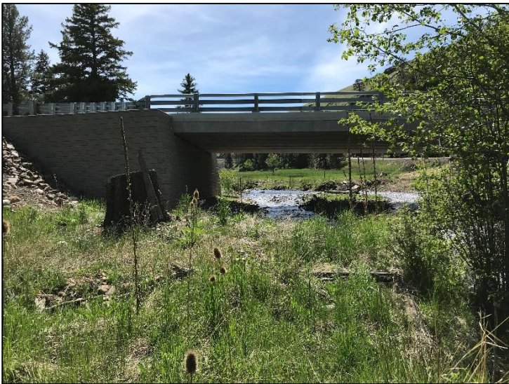
Photo 1: Top left: standing downstream of double culvert (2018). At high flow water velocity high enough to preclude fish passage and at low flow water depth through culverts is too shallow to allow fish passage. Top right: new bridge following completion of project with improved fish passage (2019) and bottom left (2021)
