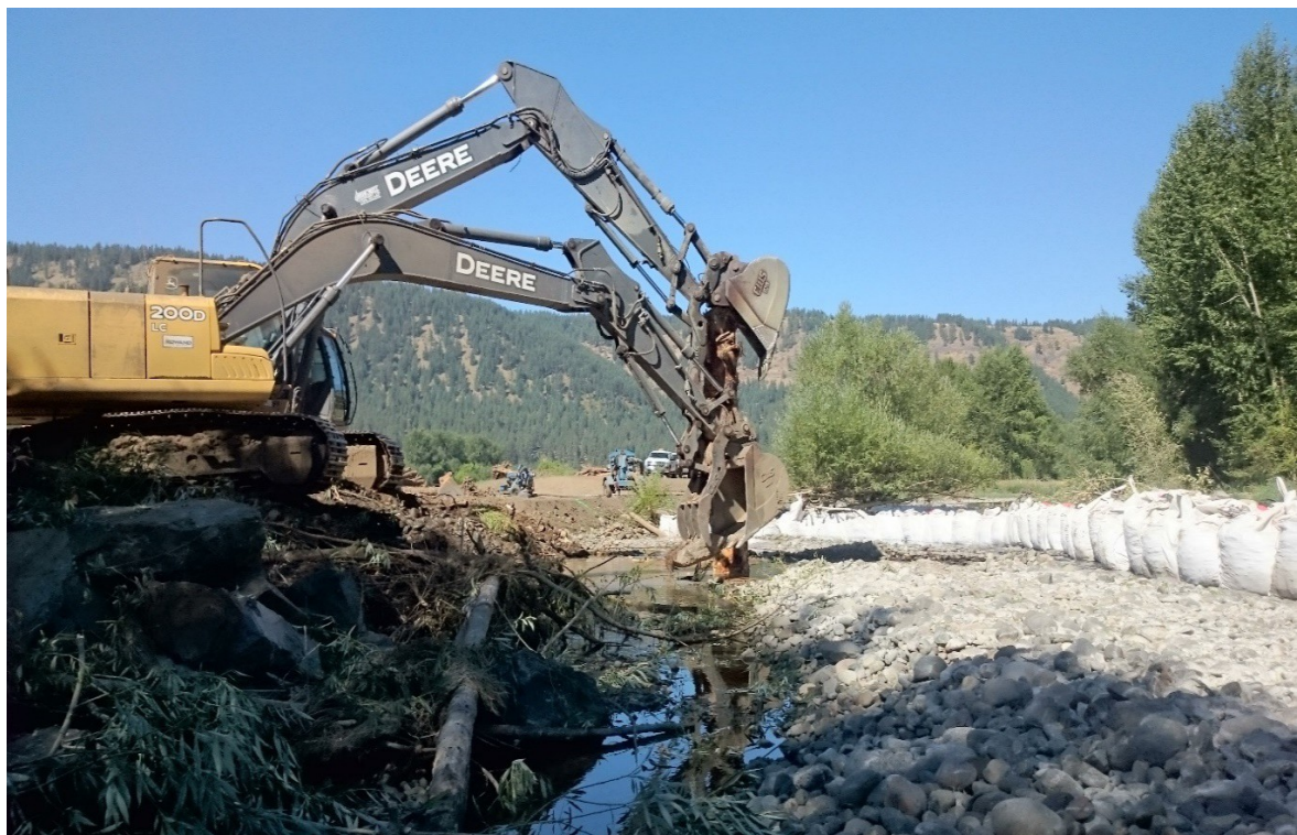
Figure 16. Construction of Wallowa-Baker Habitat Restoration Project mainstem habitat structure 8, at the inlet of Side Channels A and B, July 31, 2017.
