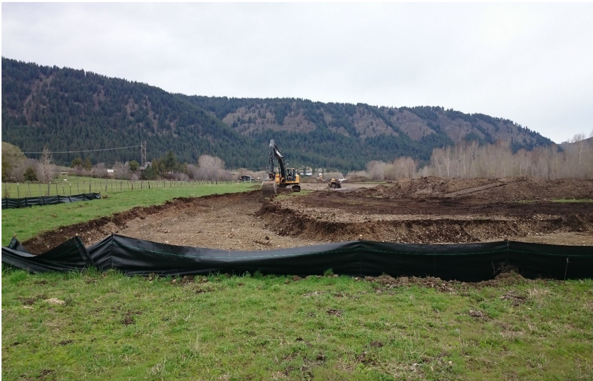
Figure 10. Floodplain and side channel construction at the Wallowa-Baker Habitat Restoration Project, April 12, 2017.
