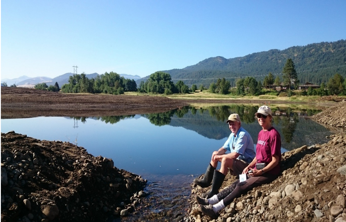
Figure 19. Landowners John and Tarrah Baker during Wallowa-Baker project construction, July 14, 2017. “Pond” formed from groundwater and irrigation run off from adjacent landowner.
