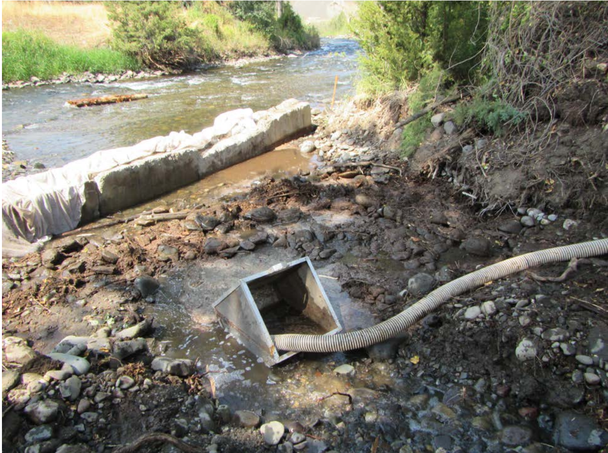
Figure 8. Sediment pump with 4 inch hose and fish screen, and Eco block isolation being implemented at the bottom of the bypass channel upon dewatering following construction.
