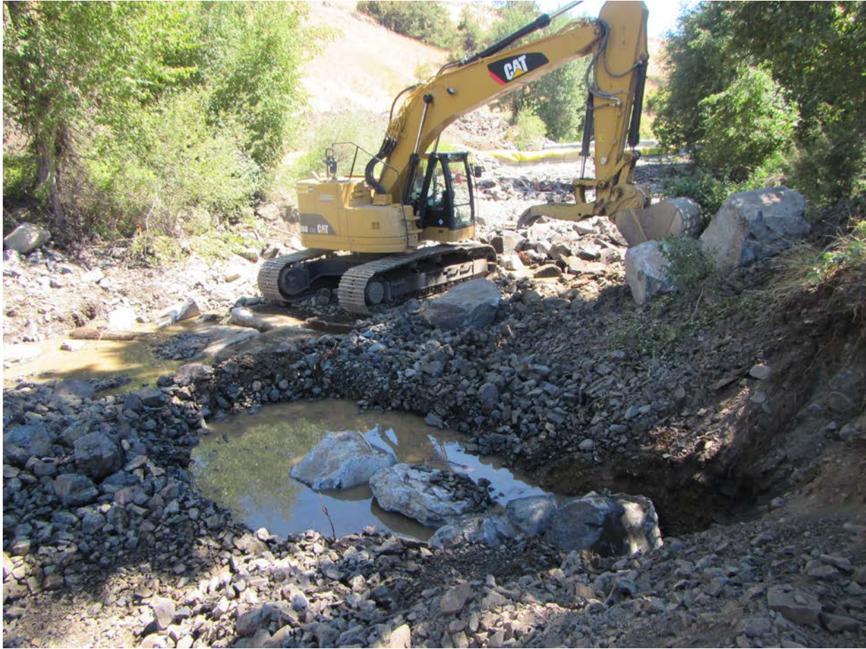
Figure 4. Contractor installing boulders to build one of eight rock weirs to maintain grade throughout the project reach.
