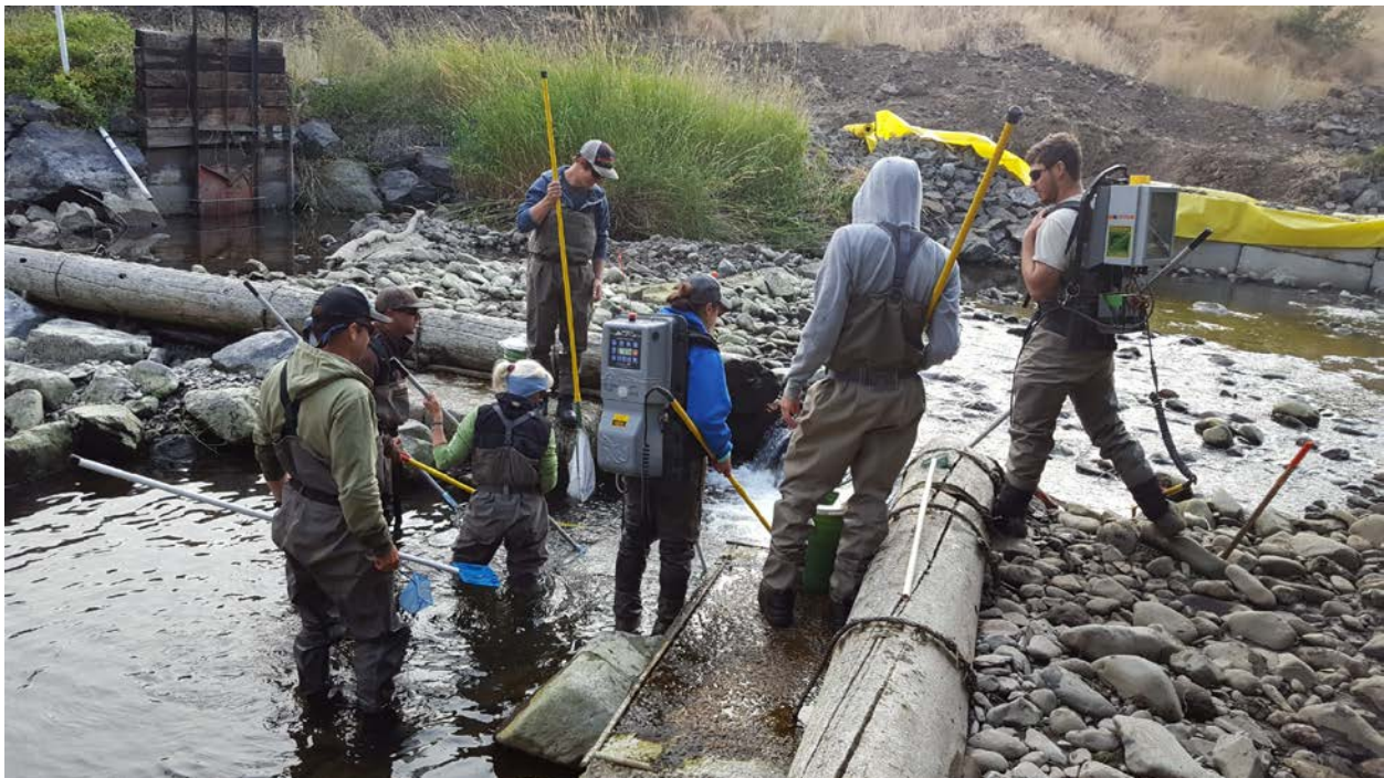
Figure 7. NPT, ODFW, and GRMW staff conducting the fish salvage in the main channel prior to construction.
