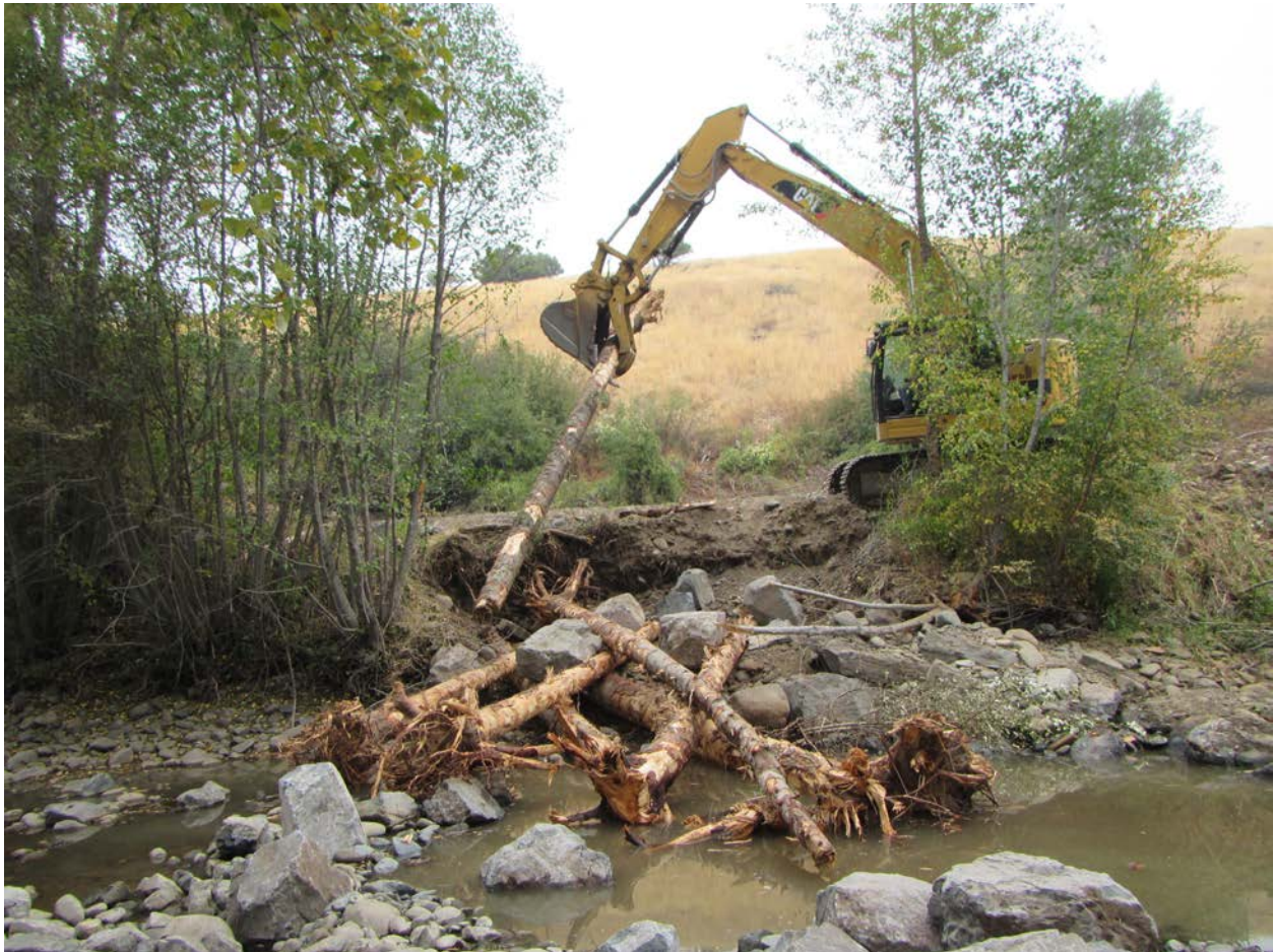
Figure 5. Contractor installing one of eight large wood structures within the project footprint.
