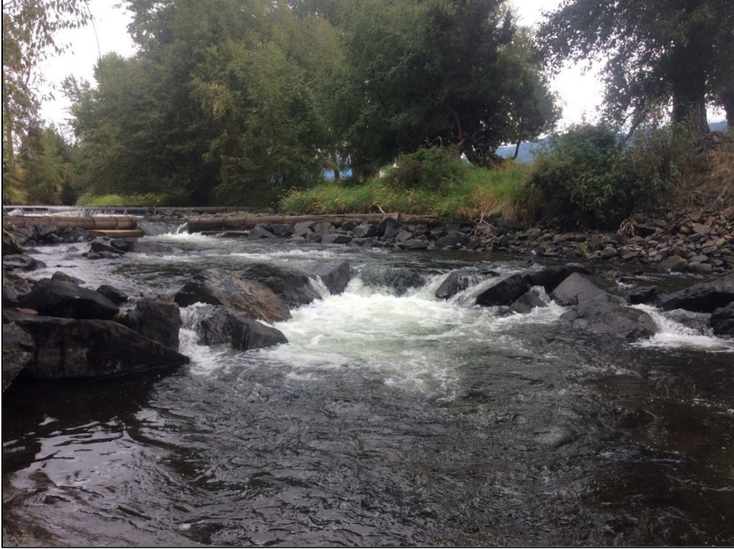
Photo 6. May 8, 2017 photo point #2 (before) from river right looking upstream through diversion, mid-project.
