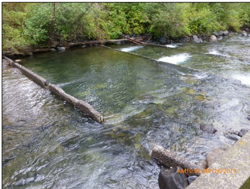
Photo 2: Standing at the point of diversion looking downstream. Part of the top concrete wall has broken off as can be seen in the foreground.
