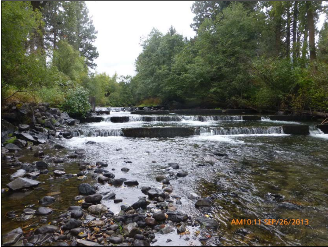
Photo 1: This photo is taken from below the fishway and diversion for the Sheep Ridge irrigation ditch. The bottom 3 walls are made of concrete, are deteriorating, and do not meet fish passage criteria as currently applied. The most upstream structure is the diversion, made of wood and as flow declines fish passage becomes more difficult.
