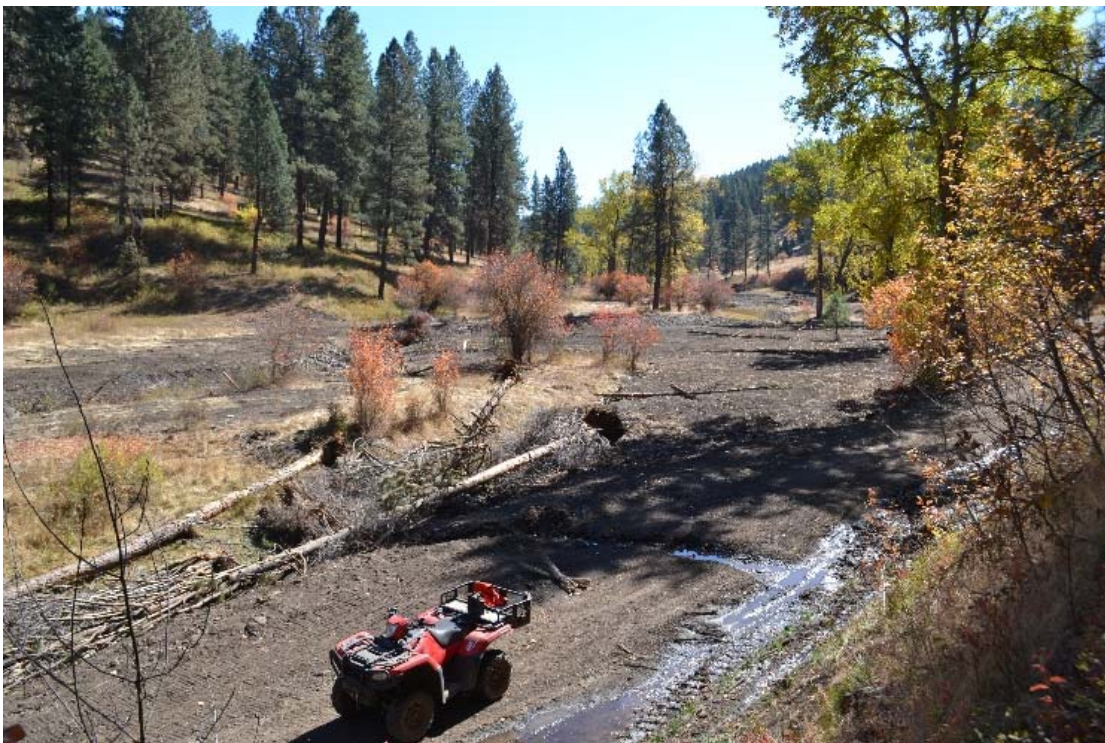
Pre-project-- road grade collecting hillside cold seeps. Pre-project channel segment converted into alcove with hillside spring connected.
