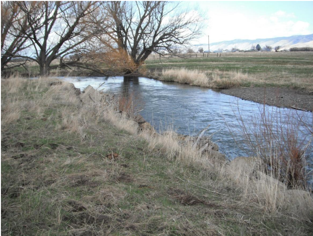
Photo 15. Eroded banks, mid-project, prior to construction.
