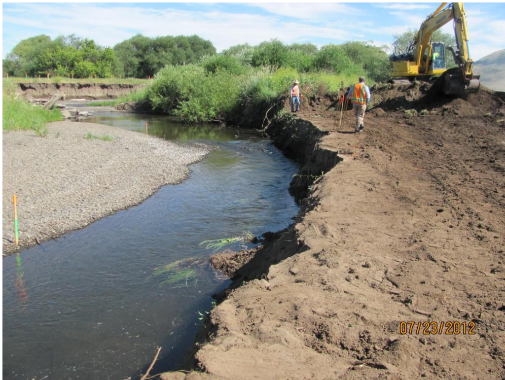
Photo 13. Vertical Banks prior to construction re-sloping and setback.
