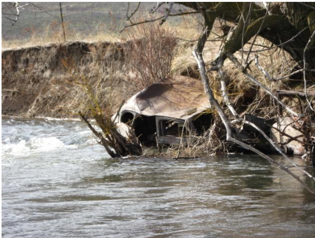
Photo 1. Vertical banks and car body “bank stabilization” pre-construction.
