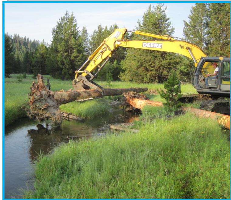
Construction of large woody debris/boulder structures is a vital prescription for improving fish habitat and stream health.
